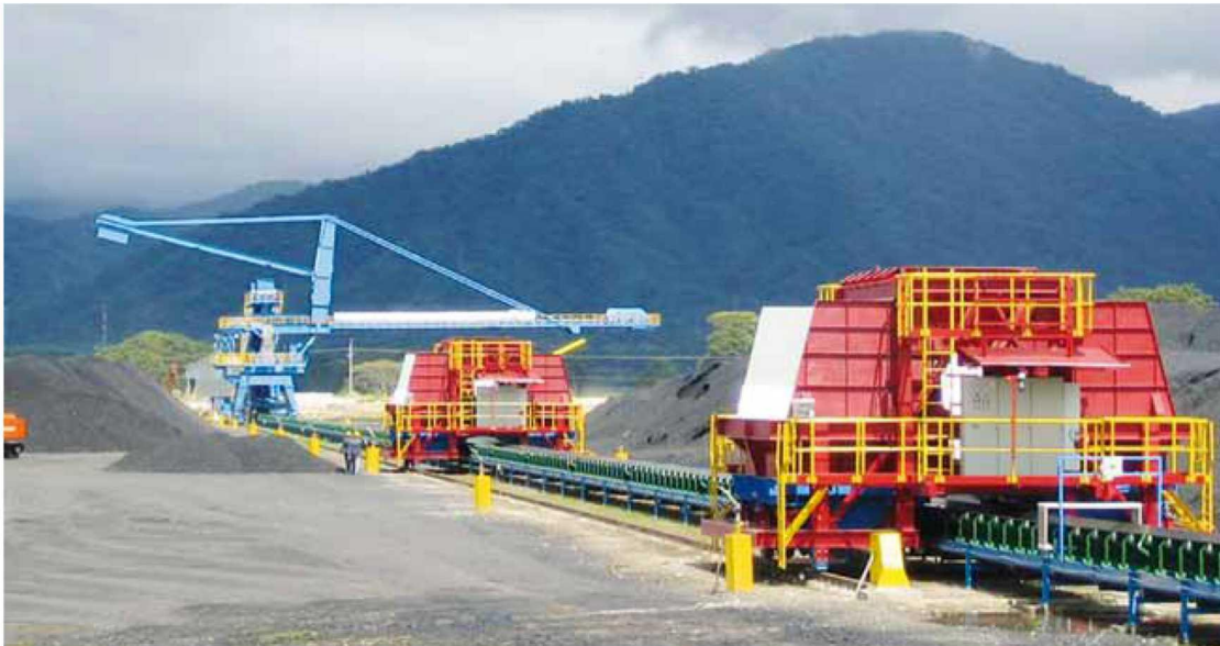
Mineral deposits conveyor
